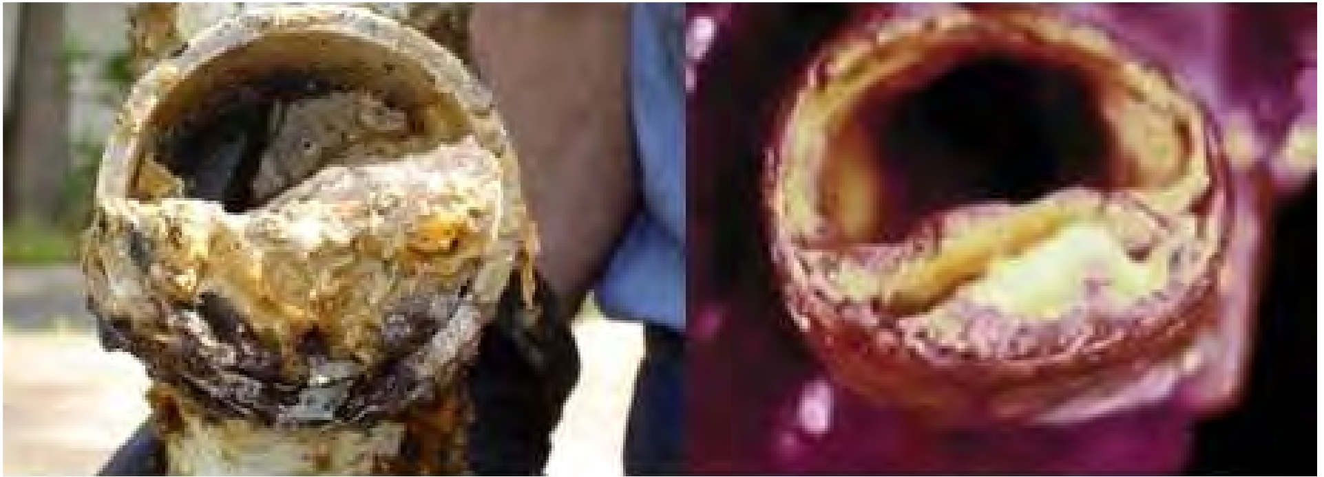
A clogged sewer
